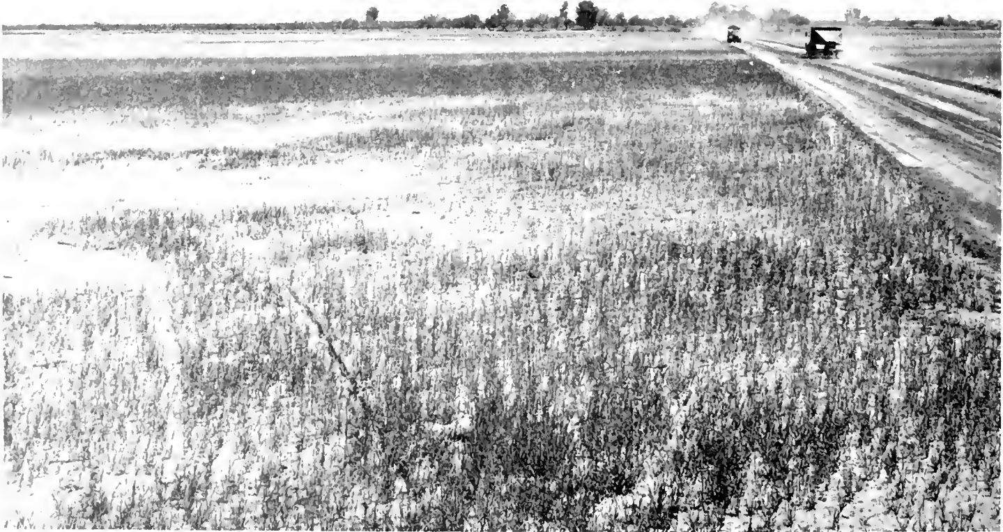
UPPER Portion of site showing completed grading and sprouting of planted cover crop. LOWER View of completed grading and start of planted cover crop.
